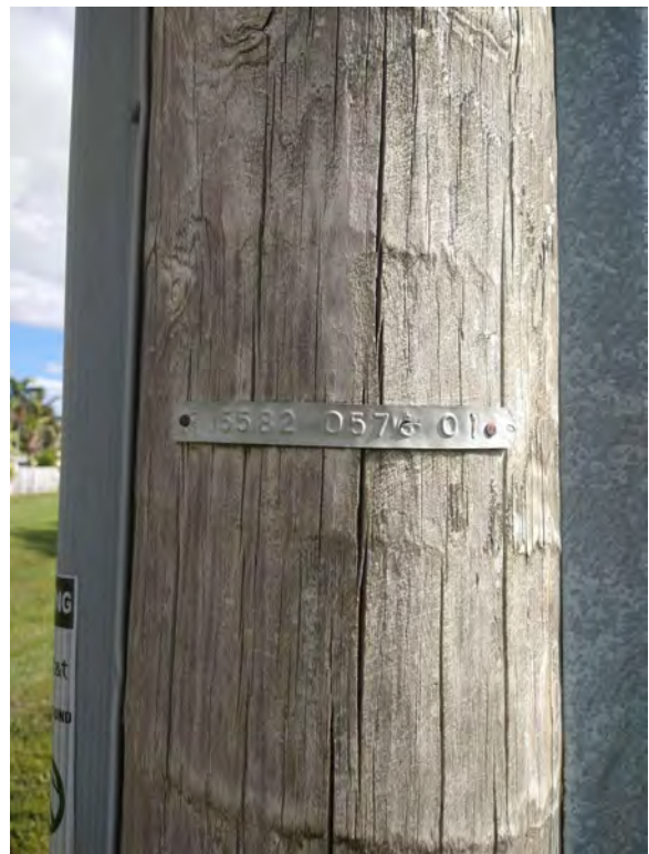
ON 27 ST. 1 ST POLE EAST OF 124 AVE 04/11/2022
