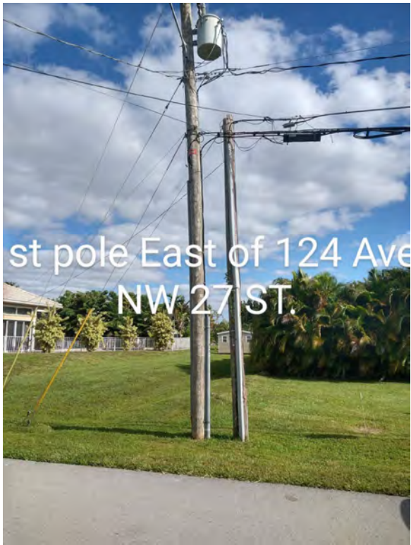
ON 27 ST. 1 ST POLE EAST OF 124 AVE 04/11/2022
