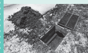
(Top) It is important to check underneath drainage grates for the accumulation of sediment, trash or debris. Pipe openings should be completely visible and free of any obstructions. (Center) It is always easier and less costly to remove any trash or build-up at this point – BEFORE it is carried further into the underground piping system. (Bottom) The removal of excess sediment will allow the structure to operate at its peak efficiency. Remember to properly dispose of the excess material and securely replace the drainage grates.
